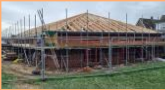
Roof going on new Memorial Playing Field Pavilion. Finish now scheduled for May—Page 25.
