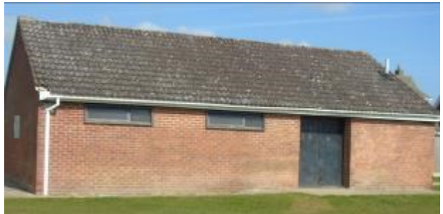
The existing not fit for purpose pavilion on the Memorial Playing Field.
